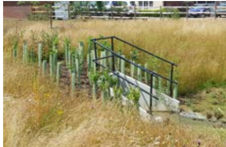
ILLUSTRATIVE EXAMPLE YOUNG NATIVE SHRUB PLANTING BEHIND HEADWALLS WHICH TO DISCOURAGE ACCESS
